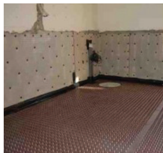
Installation of flood protection system - Newton 508 Mesh applied to walls and Newton 520 to floors
