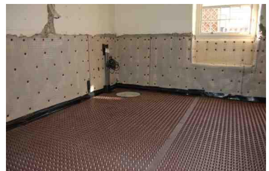
Newton Water Management System fully installed
