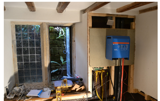
Temporary installation of the Newton Victron Quattro Inverter while other internal works were being finished
