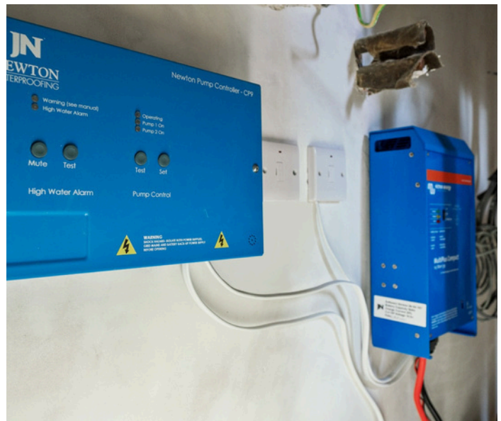
A control panel and power inverter provide complete peace of mind.
