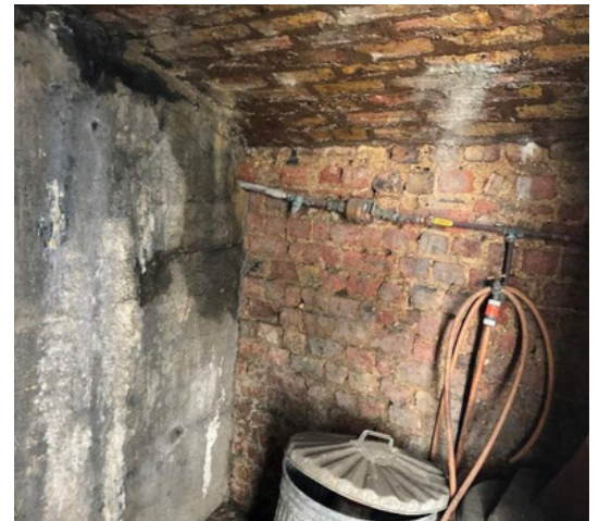
The existing basement vaults were extremely damp.
