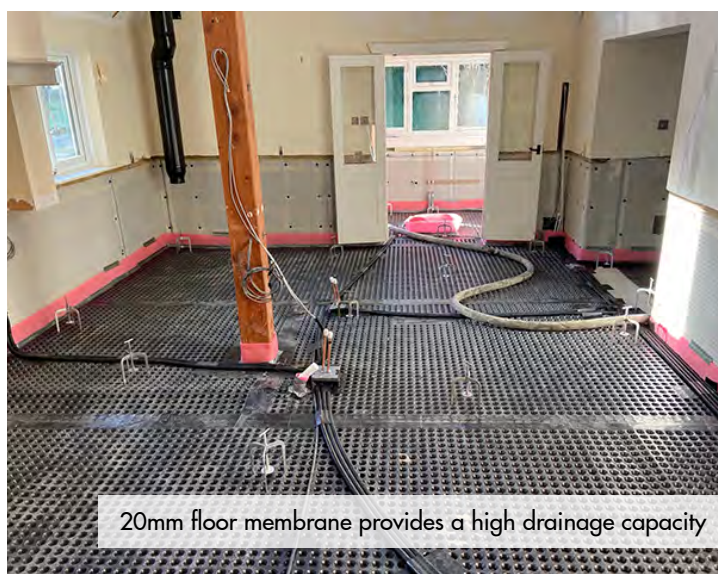
The CDM System was installed throughout the ground floor
